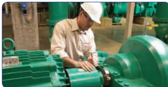
The correct choice of surface coatings can help to reduce losses from corrosion in the water industry
