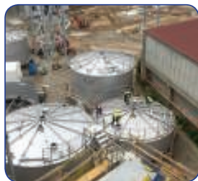
BUTTING supplied vessels and pipework for this starch plant
